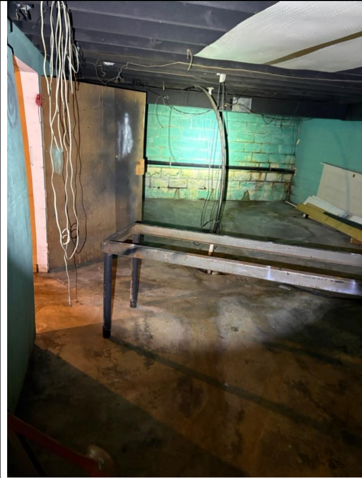
Evidence of water intrusion and standing water in basement.
