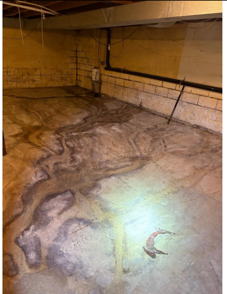
Evidence of standing water and possibly sewage collection stains on floor.
