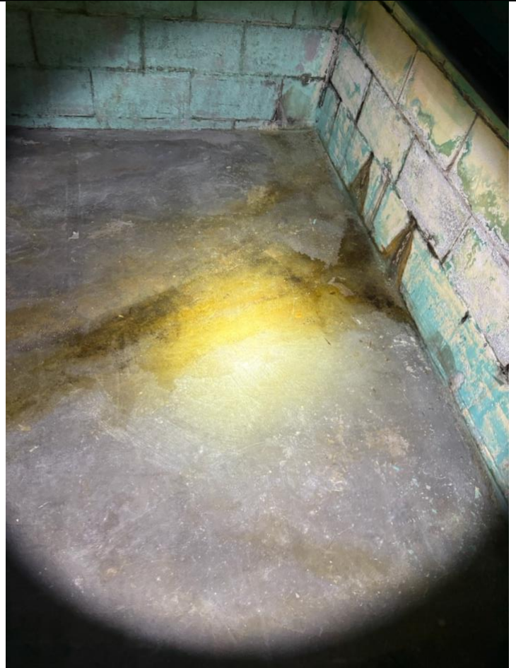
Evidence of water intrusion through block foundation walls.
