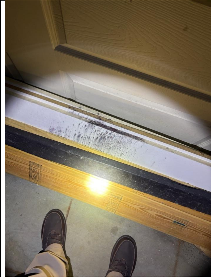
Fungal growth on stored building materials.
